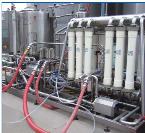
Oenoflow HS-12A System at Chilean winery
